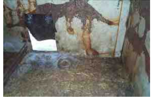
8-21. No bedding, rusted dog enclosure 3.1(c)(1)(i); 3.3(a)
