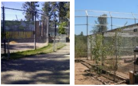
Compliant big cat fencing
