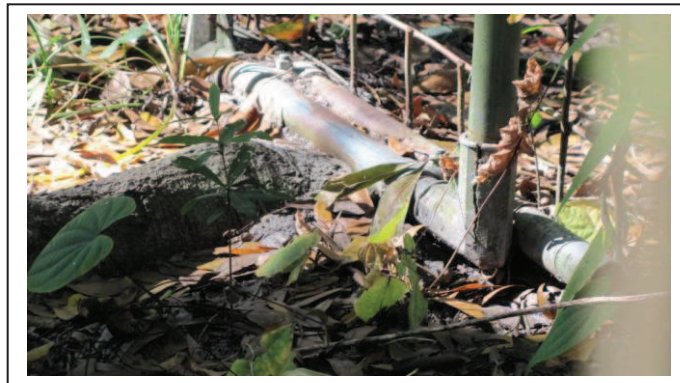
Support pole cracking
