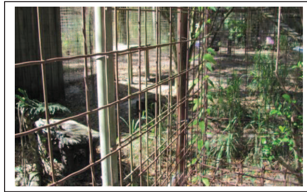
Surface rust on support pole
