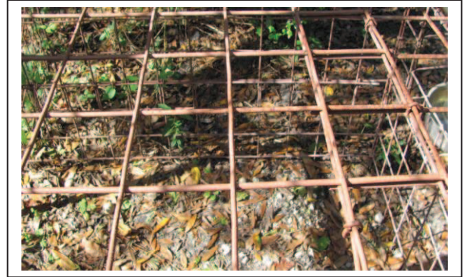
Rusted/pitted wire upper panel
